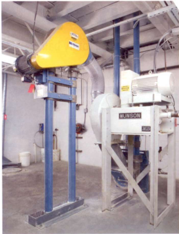
A side view of the attrition mill. The yellow box houses the drive for the mill's 14.9-kW motor
