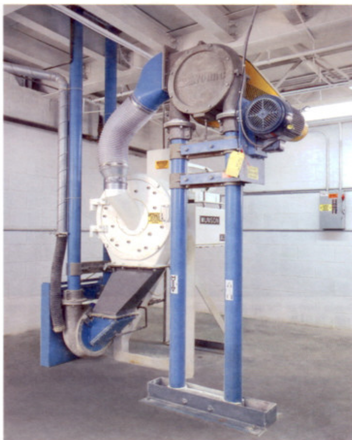
Fine powders are processed in this attrition mill (centre left) and pneumatically conveyed to the packaging area via the blue tube at the left
