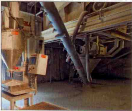
Screw conveyor transports blend.
