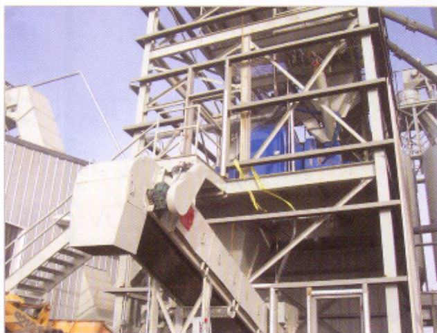
The rotary batch mixer totally evacuates blended material, which is gravity discharged into this 4082 kg capacity surge bin.
