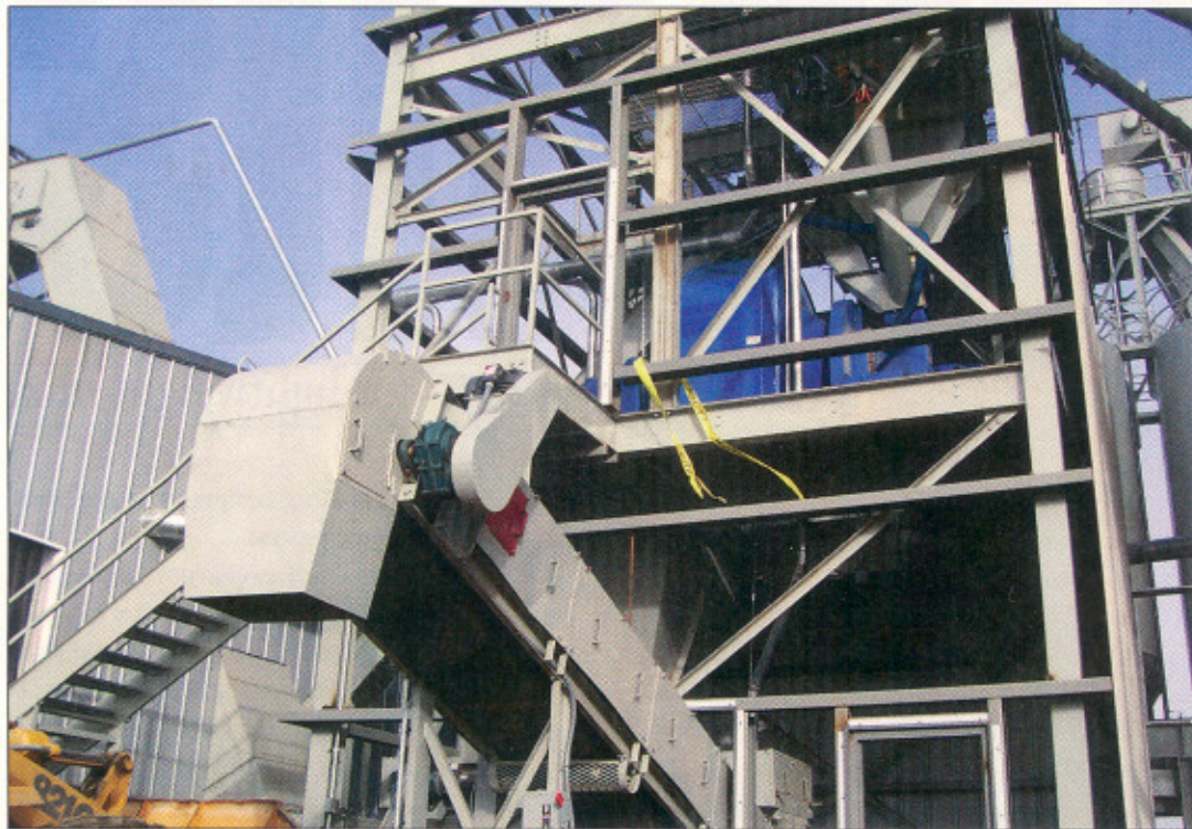
The rotary batch mixer totally evacuates blended material, which is gravity-discharged into this 9000-pound capacity surge bin.
