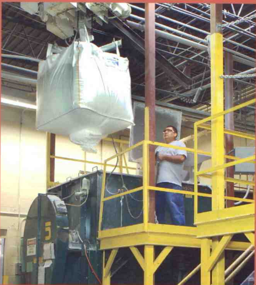
Bulk bags containing cellulose ride on a track that is angled to optimize the use of floor space.
