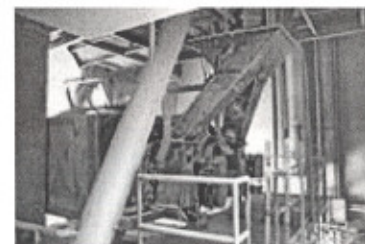
Raw materials are discharged from the scales above and flow through the diverter gate (center, rear) into mixer no. 1 or no. 2. The pipe in the foreground is not integral to the mixing operation but is used if material has to be transferred from one storage bin to another.
