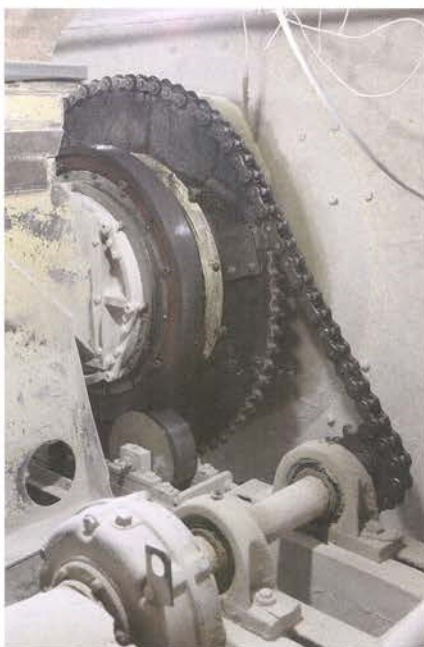
To prolong the batch mixer’s service life, Anchor Glass performs scheduled maintenance to replace the equipment’s limited wear parts.
