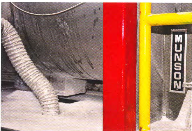
Material discharges through the bottom port of the blender into the hopper and filling machine on the floor below.
